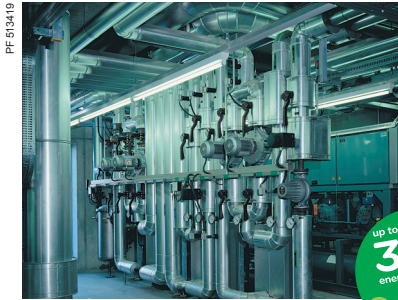
ATV12 controlling a pumping station
