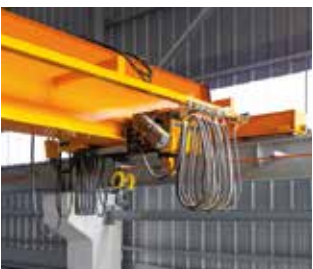
GRAVITATIONAL HANDLING EQUIPMENT
